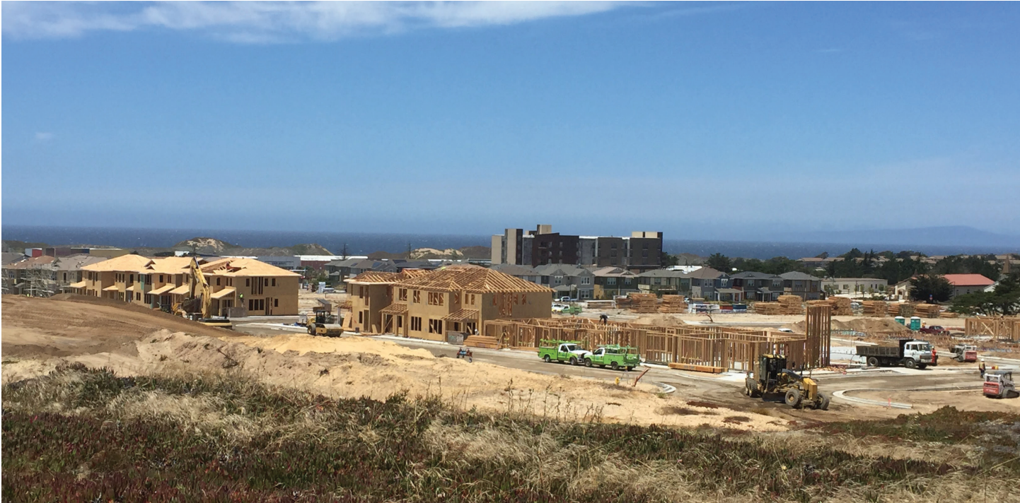
View above the Dunes Housing development construction and Marriott Spring Hill Suites Hotel near completion.
