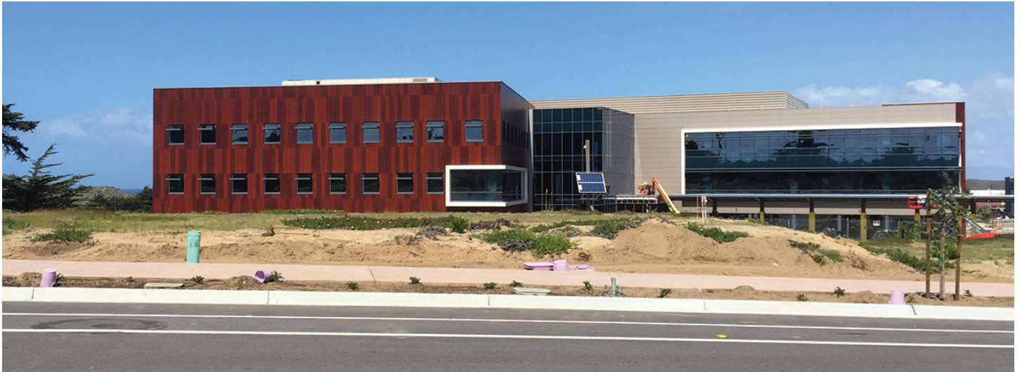
The new joint DoD/VA Monterey Bay Health Care Clinic is expected to be completed and open in Spring 2017
